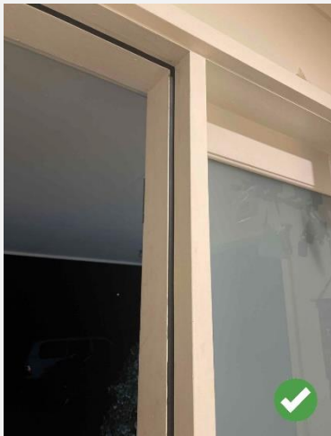
Figure 4: Post-installation photo showing weather seals on two sides of door frame (additional photo required to show whole of door frame is sealed)
