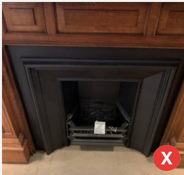
Figure 5: Interwar period fireplace which fully seals - front view
